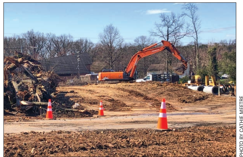
Construction equipment on the move at the site for condos for age 55+ on Greenbelt Road, near the Armory
