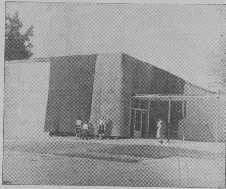
CURTAIN GOING UP! New GCS building as of last Saturday before the windows were put in.
