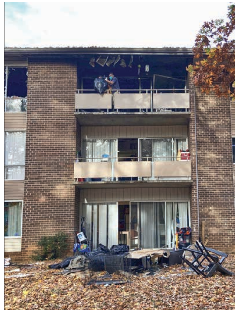
Workers begin removing debris from the top floor apartment and repairing water damage in the apartment below in the afternoon after the fire.
