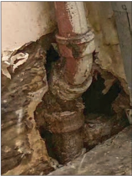
A rusted-through laundry drain pipe, photographed in September 2023
