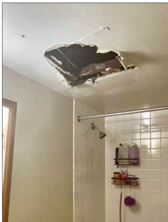
A water-damaged bathroom ceiling in a Charlestowne North apartment
