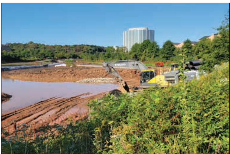
Work is underway on the stormwater retention pond at Ora Glen Drive and Hanover Parkway. The retrofit of the pond will allow for improved removal of pollutants from storm runoff before releasing it into local waterways.
