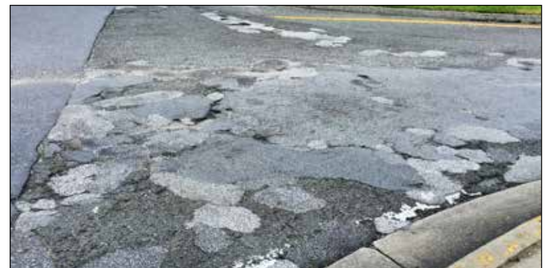
Efforts to get the state to fix the intersection at Kenilworth and Edmonston results in a rough patchwork of asphalt.
