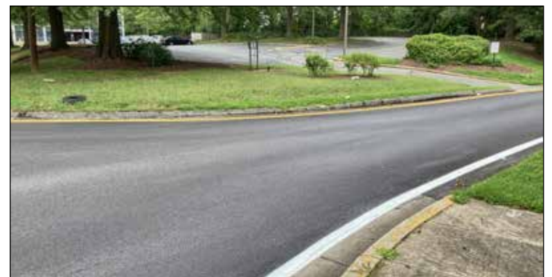
With a complete resurfacing, the ramp now gives smooth sailing all the way.
