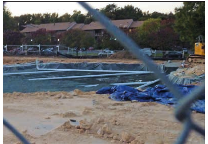
Construction crews pull up some of the asphalt at ERHS to put in a filtration system, in order to create a green parking lot.
