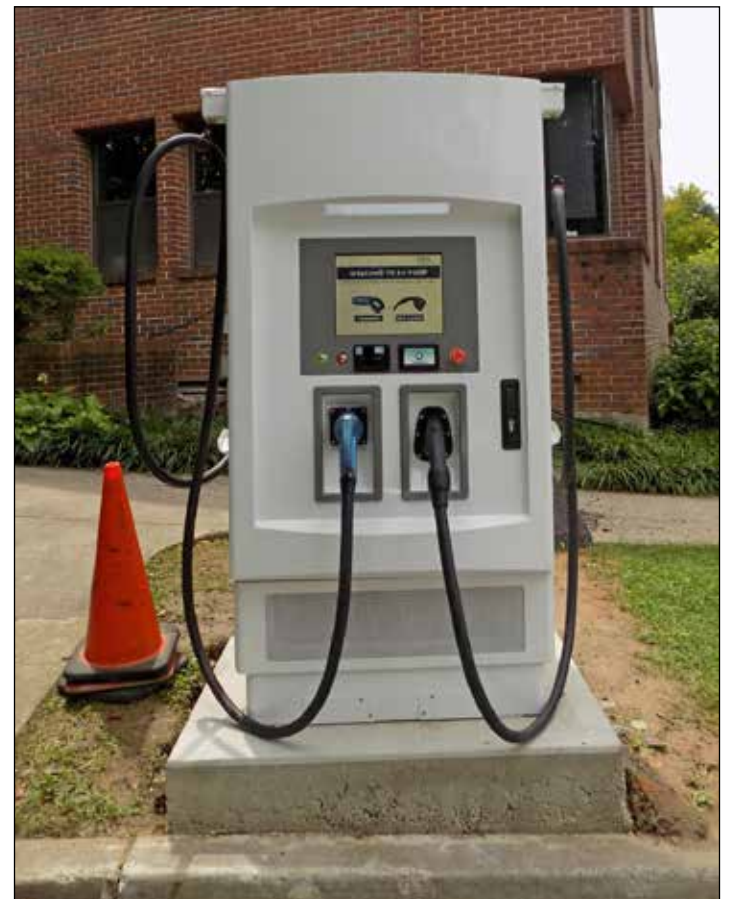
A new electrical charging station is located next to the Municipal Building
