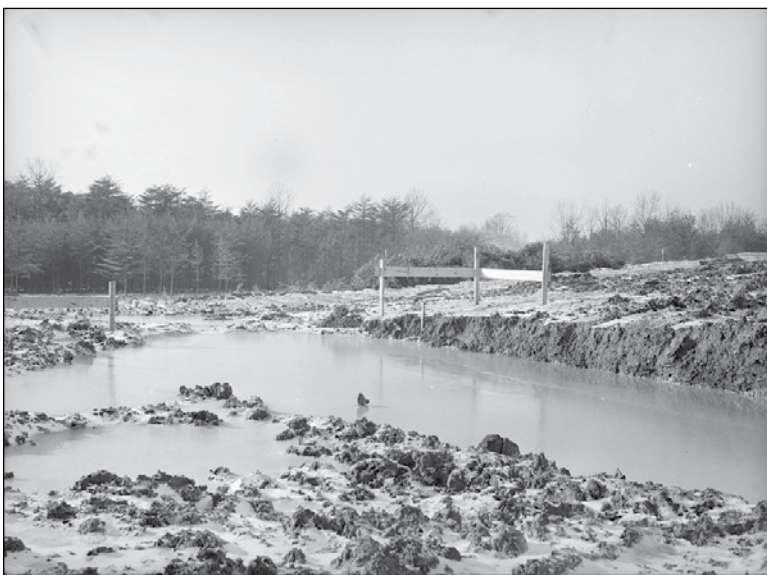
Flooded and frozen foundations during the winter of 1935-1936
