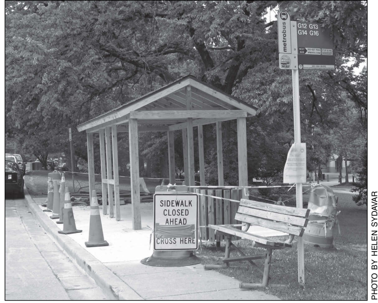
Progress is being made on the construction of a new bus shelter at Roosevelt Center. Service has been unaffected. Improvements are made possible through a Metro partnership with the City of Greenbelt.
