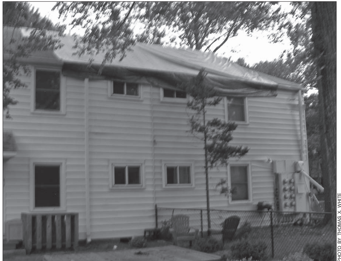
A view of the burned end of 61 Court Ridge where all units are currently uninhabitable due to fire and water damage from the September 22 electrical fire.
