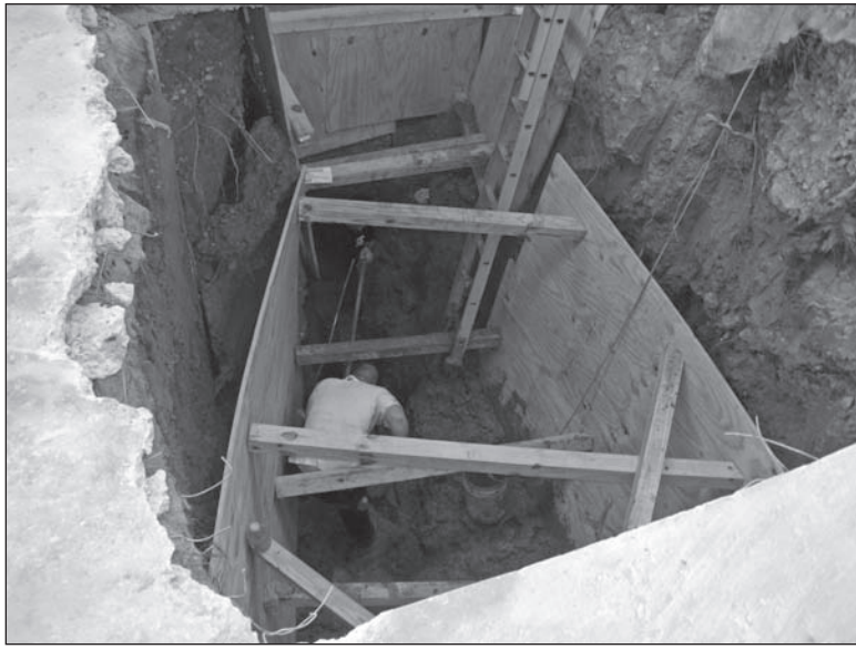
The big dig – The sidewalk in front Greenbelt Cleaners was dug up to fix a leaking sewage pipe. Much of the excavation work had to be done by hand with shovels and buckets.
