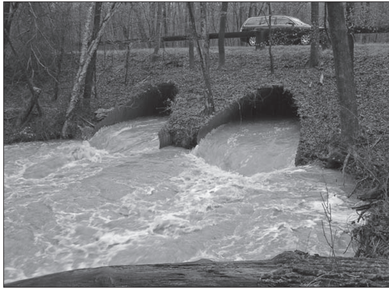
Runoff from a 30-minute storm overloads Still Creek stream capacity. High water tears away at the banks and cuts deeper down into the streambed carrying away huge quantities of soil.
