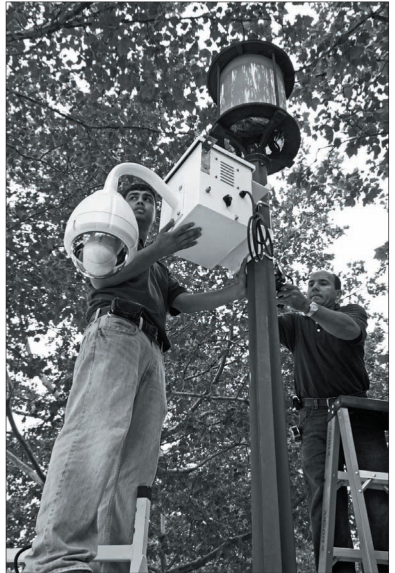
Avrio Systems contractors work to install one of the new video security cameras at the Roosevelt Center. When the work is completed there will be one stationary camera and three with pan/tilt/zoom capability. According to City Manager Mike McLaughlin, the cameras are expected to be operational in about one week.
