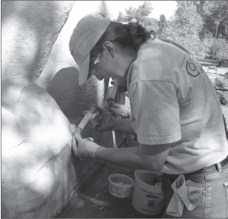
A member of the conservation team cleans and repairs the 70-year-old Mother and Child statue in Roosevelt Center and the friezes on the Community Center. Above, the worker injects sealer to fill cracks. —photos courtesy of Conservation Solutions
