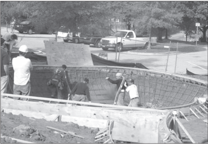
The recreation department reports that work on the skate park continues. Fine grading and installation of forms is almost complete. Installation of rebar in the "bowls" began this week. Depending on weather and a successful inspection by the county, shot-crete on the bowls will begin this week.
