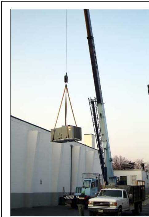
Stunned to see a huge crane towering over Roosevelt Center at 6:30 a.m. Saturday, March 19 local photographer Tom Carter grabbed his camera to snap this photo just as the new air-conditioner for the movie theater was being hoisted onto the roof. Cool.
