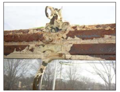
Lead paint is pushed off surface of the metal by rusting steel. Hardware is all bronze and should not be painted.
