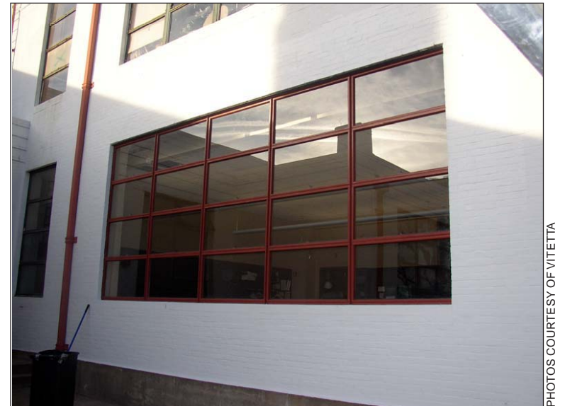
Restored window with replaced concealed lintel behind the white painted brick above the window.
