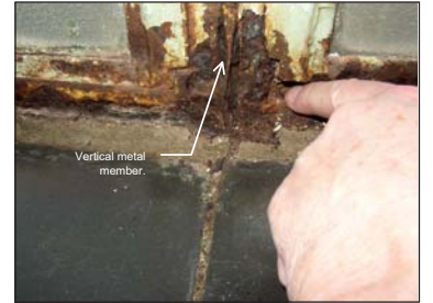
Metal has completely rusted away at bottom (vertical structural member no longer anchored at sill).
