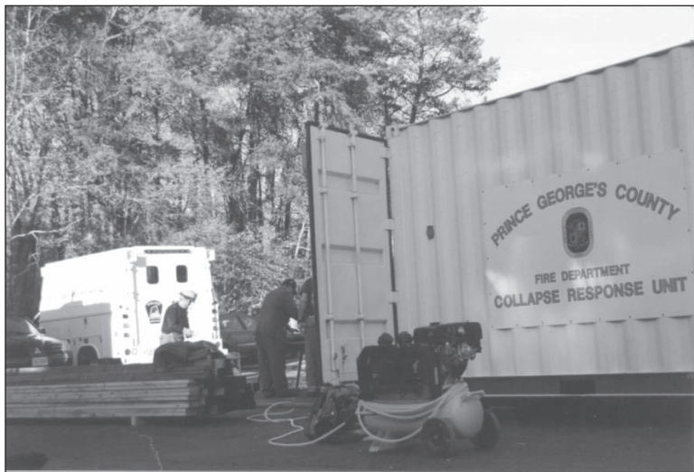
A huge flatbed truck dropped this Collapse Response Unit at the site. It's a self-contained workshop with materials to shore up a fire-damaged building.
