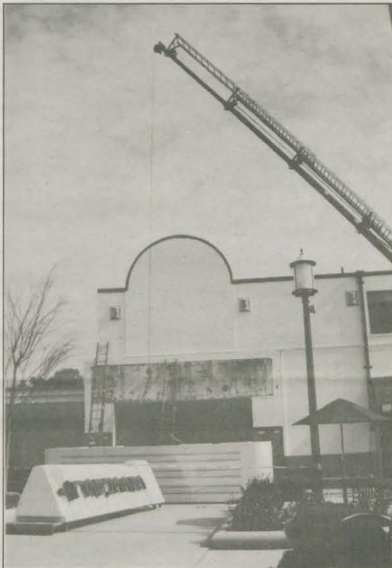
The crane places the signs in front of the theater, where they sat for several hours. photo by Steve Catterton
