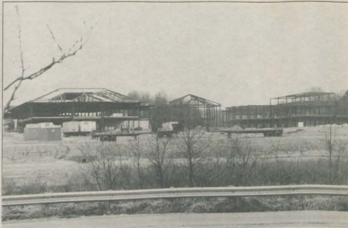
Construction continues on the four-building USDA headquarters complex on Sunnyside Avenue as this late January photo shows. -photo by Mary Moien
