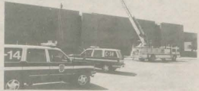
Firefighters were called to Eleanor Roosevelt High School last week when smoke was discovered in the library on the second floor. A malfunctioning air handler was the cause and was shut down. No damage occurred. —photo by Tom Carter
