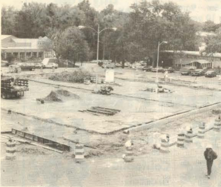
West parking lot shows effects of demolition of former islands and removal of trees. New curbing shows at right edge of picture. —photo by J Henson
