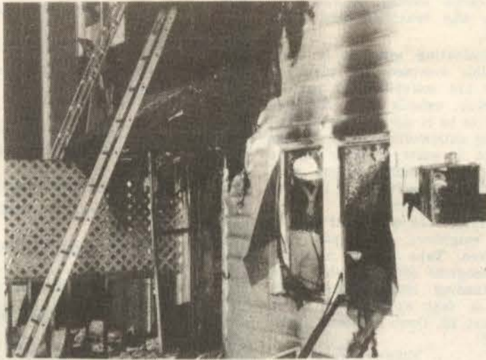
An unidentified firefighter pulls down drywall to check for fire extension within the wall.
