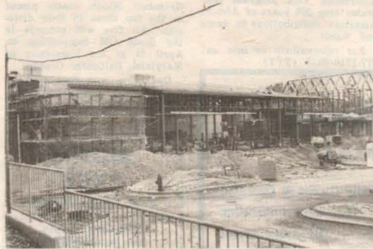
The front of the new elementary school on Ridge Road begins to take form with the completion of the steel structure and placement of base roofing. Construction of masonry walls is underway. —photo by J. Henson
