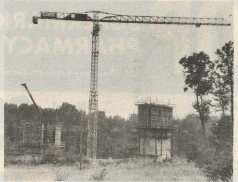
Reinforced concrete towers are erected as the first phase of construction of the new Federal Courthouse for the Southern Maryland Region on Cherrywood Lane opposite Capital Office Park. —photo by J Henson
