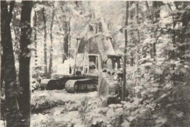
The backhoe places rocks in the stream next to Braden Field. The rocks will slow th stream's flow.
