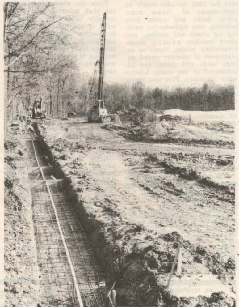
Concrete footings are ready to be poured as pile driver (crane) works in background at the new elementary school site. Groundbreaking ceremonies took place Saturday, April 25. — photos by J. Henson
