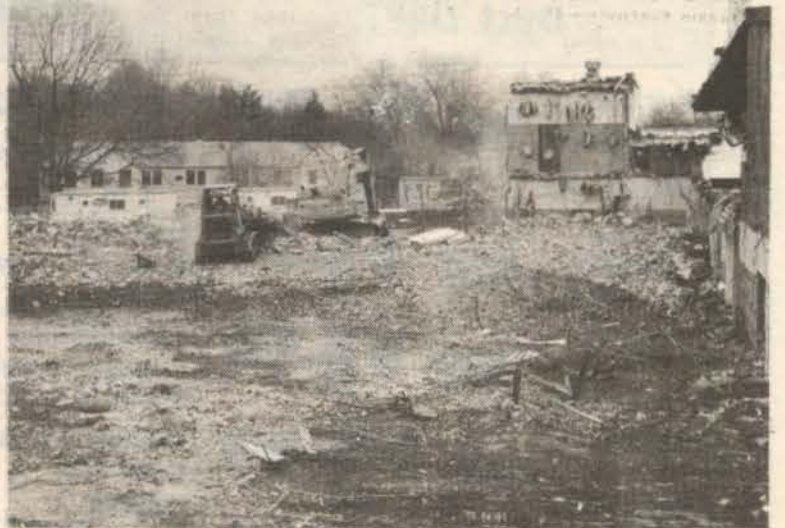
Homes on Laurel Hill Road have a changed view as bulldozer cleans up the rubble from partly demolished North End School.
