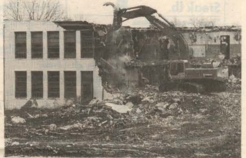
North End School is attacked and demolished by a large machine. All that remains is rubble which is rapidly being hauled away.
