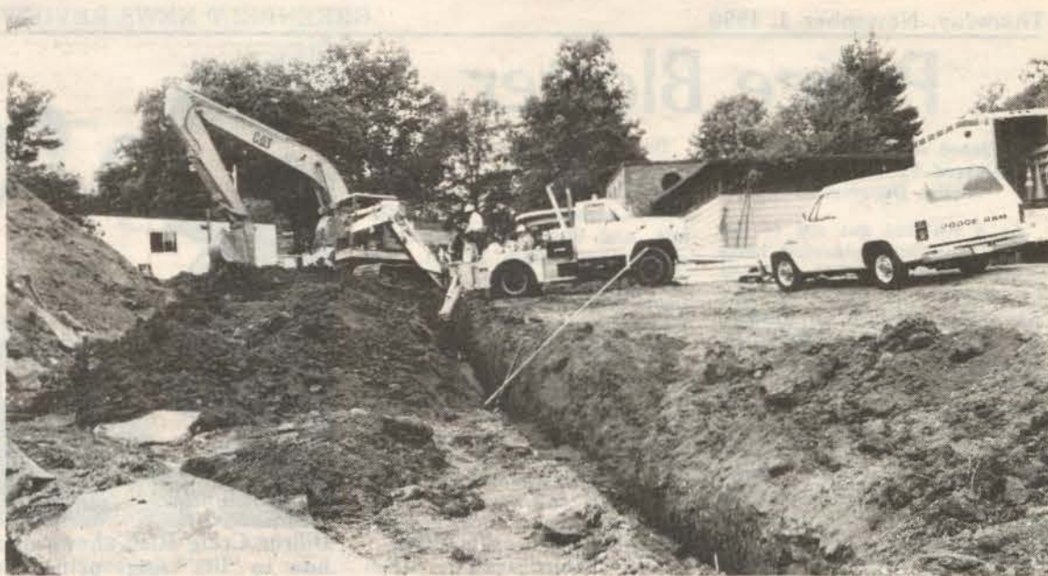
Work is underway at the construction site of the indoor pool. The old bathhouse of the outdoor pool is at the upper right behind the trucks. — photo by J. Henson
