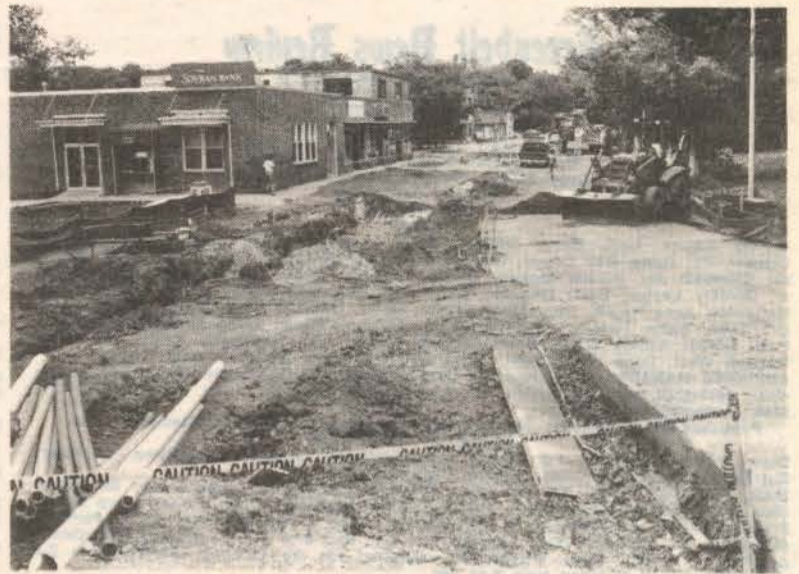
Centerway and the adjacent sidewalk are torn up during renovation. — photo by J. Henson
