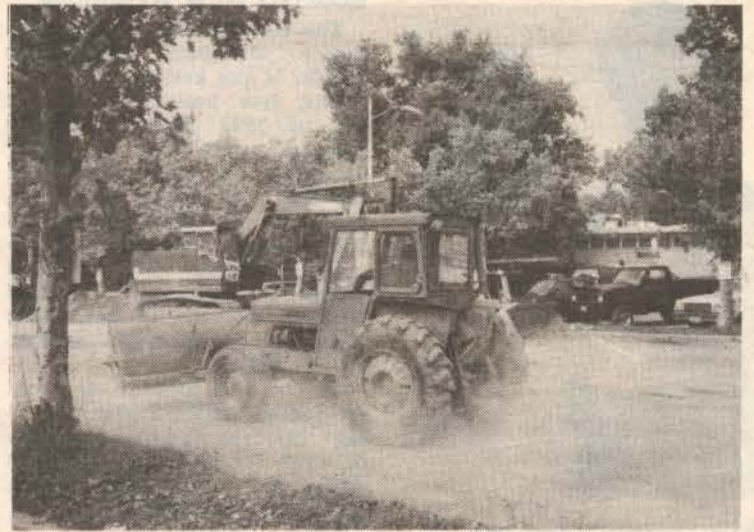
NZI keeps its word to Council, and the bulldozers rolled. Shown here, they are completing the laying of the 8-inch water line for the indoor swimming pool within four days of council's approval of the project.
