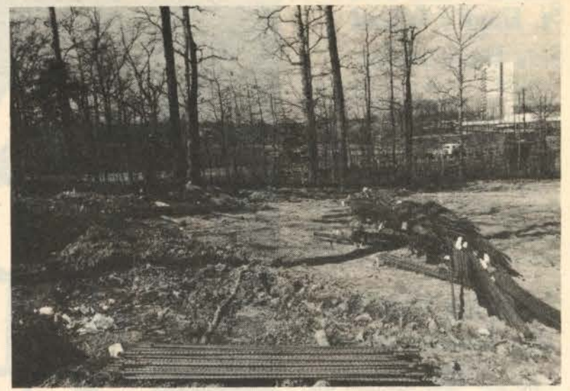
View from site cleared for new Greenbelt police station looking toward Kenilworth Avenue. The Greenbelt Hilton and Towers is visible in the background.
