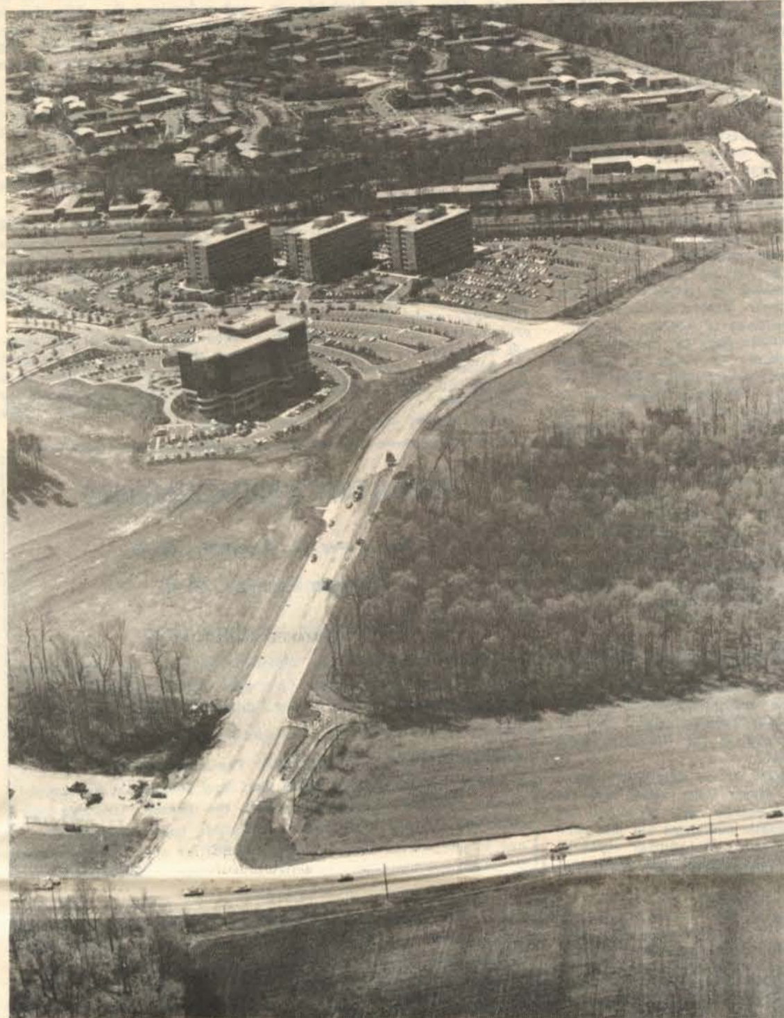
Aerial view, looking west, of the construction of Cherrywood Lane Extended from its intersection with Edmonston Road (Kenilworth Avenue) to its intersection with Ivy Lane in the Capital Office Park. Visible just beyond the office park is the Beltway, with Springhill Lake beyond. Eventually, the bridge will span the Beltway and Cherrywood and become a direct connection between Edmonston Road and Greenbelt Road (at the west end of Beltway Plaza). — photo by Bill Cornett
