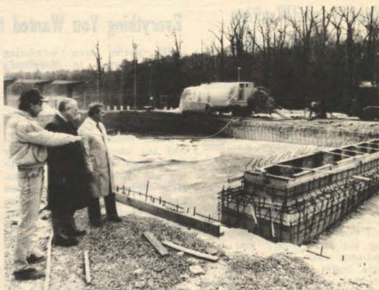
City Manager, James K. Giese, center, and Recreation Director, "Hank" Irving, right, listen as George Rogala, area Recreation Supervisor, points out construction work on the Municipal Swimming Pool being renovated by Olympic Swimming Pool Company and designed by Sullivan and Almy Associates. — photo by Nick Pergola
