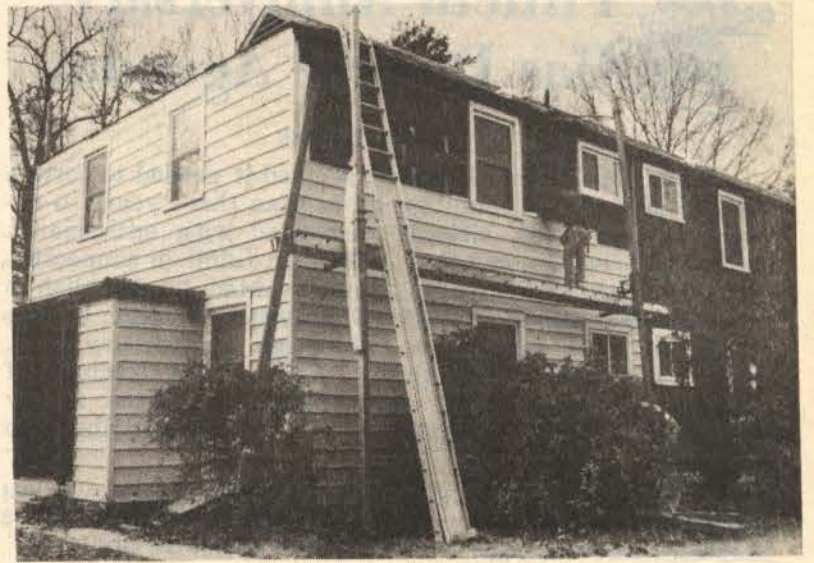
"... Deteriorated asbestos shingles on the frame homes were replaced with vinyl siding."
