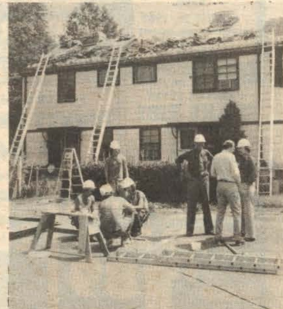
Work begins on GHI's long awaited rehabilitation program with roof replacement on 73 Court of Ridge.
