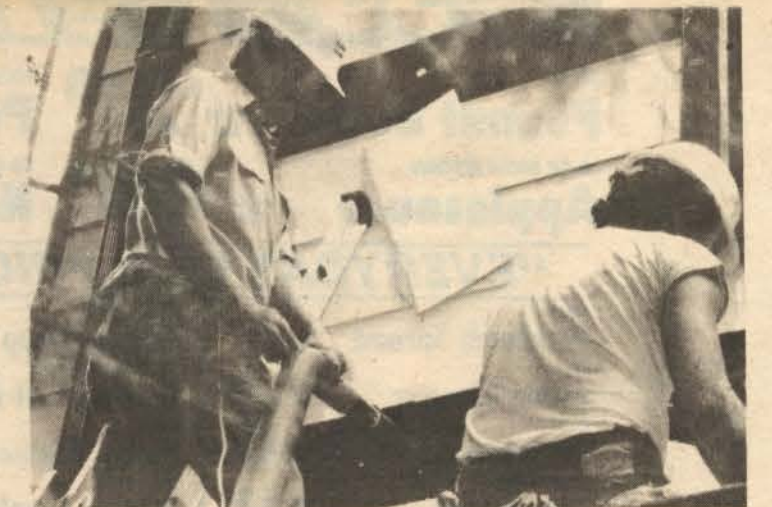
Workmen demonstrate installation of Cellin, cellulose insulation, which is blown into the outside walls through one inch holes. Bill Glass, representing the contractor, Universal, was on hand to answer questions. "No, Cellin will not burn. Yes, it is termite and varmint proof. Yes, the contractor will guarantee to fill the cavity 100%. No, there is no odor. All work will be done from the outside."
